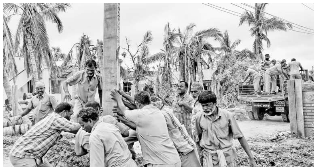
Teams of electrical workers are a common sight now across districts in the delta region. • SHAJU JOHN
